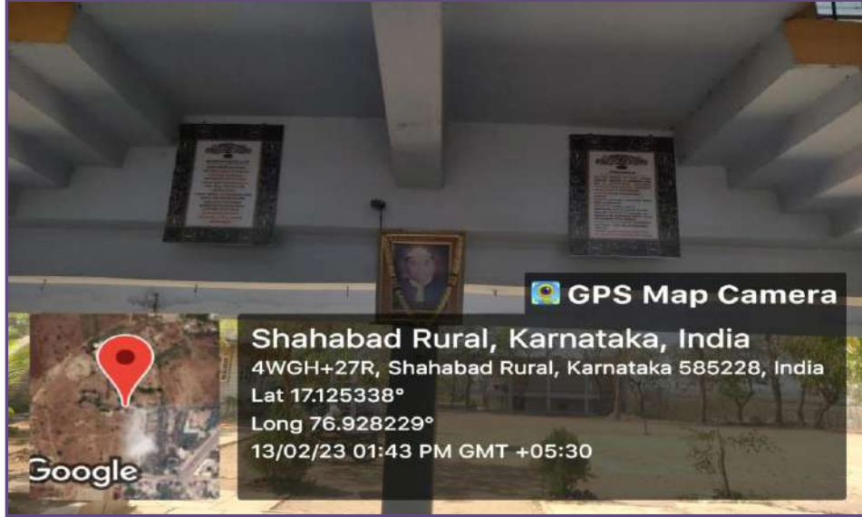
CCTV Cameras in the main entrance of the campus
